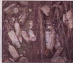
Debris in drainage ditches causes Route 17 floods.
